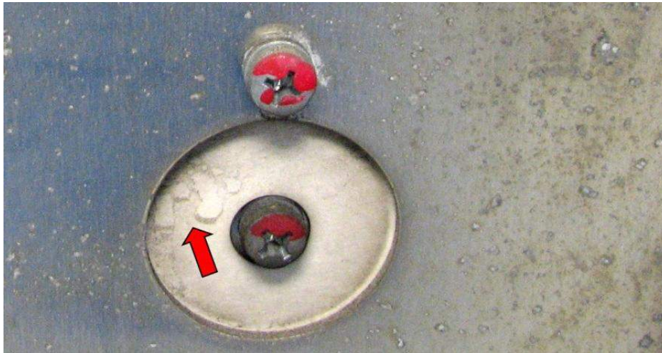
Figure 7: Evidence of liquid having been present on insulation of a DC link assembly
