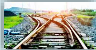
Rail Track Condition Monitoring
